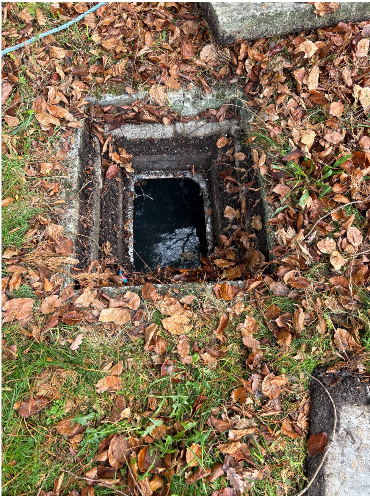
The septic tank.
